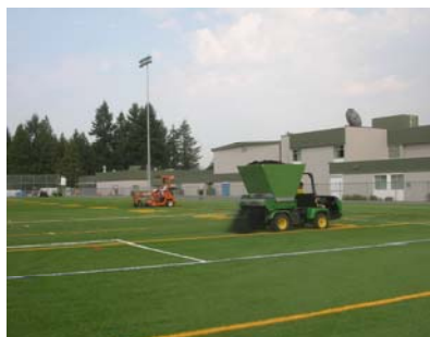
Completion was scheduled for mid-August to allow user groups to use the field for summer sports and practices
