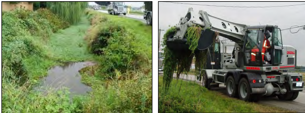
Figure 1. Vegetation growth (parrot feather) and removal using gradall in Baynes Roadside Ditch
