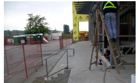
New steel handrails have been installed at the entrance of the building.
